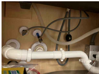
Kitchen Sink Plumbing
